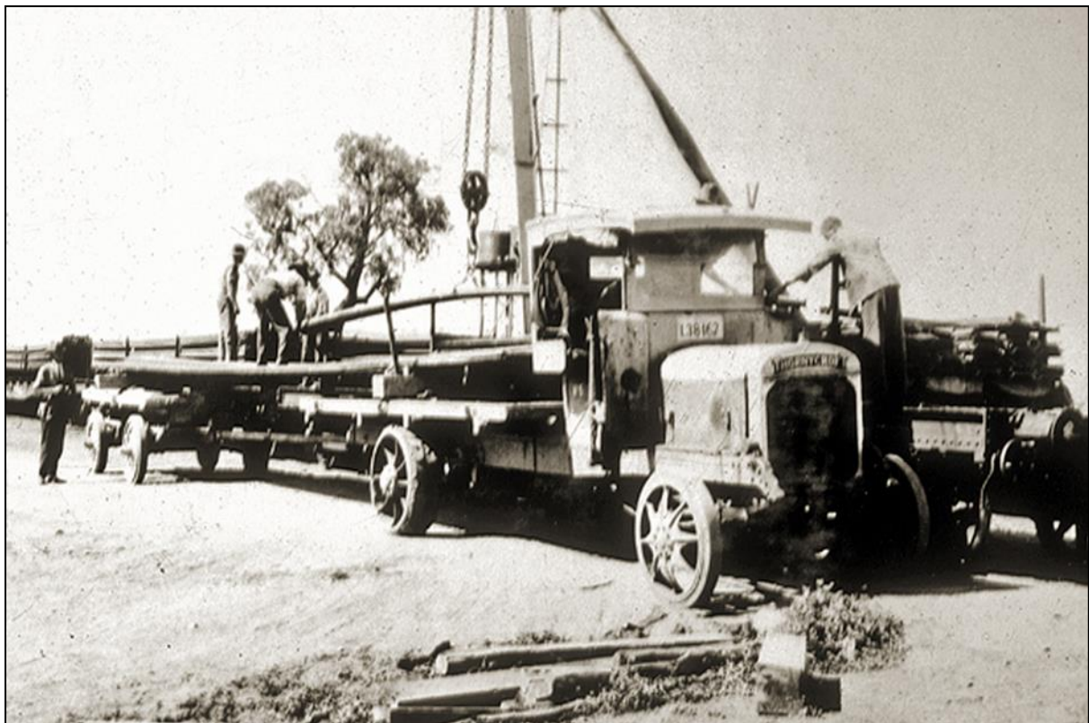
One of the ten Thornycroft Lorries being loaded. They ferried equipment from the Albury railway siding to the NSW construction site.
